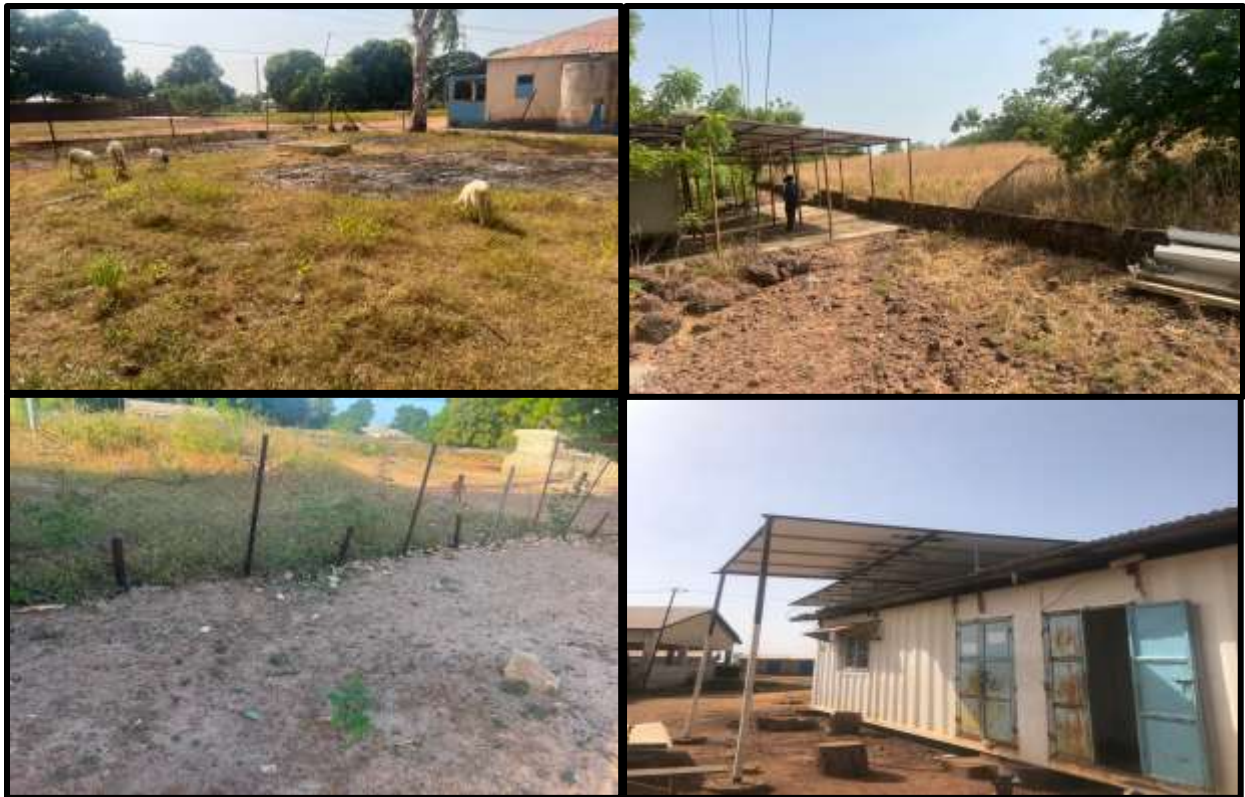
Picture 3 shows sites with perimeter fence problem
