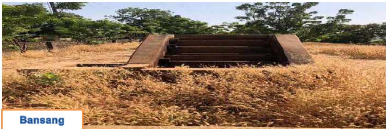
Picture 8: Abandoned aerator at Bansang Water Treatment Pant
