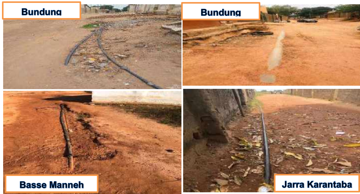
Picture 4: NAWEC’s exposed distribution pipe (top Left), main pipe (top right) in Bundung and exposed distribution pipe (Bottom left) exposed distribution pipe at Jarra Karantaba (Bottom right)
