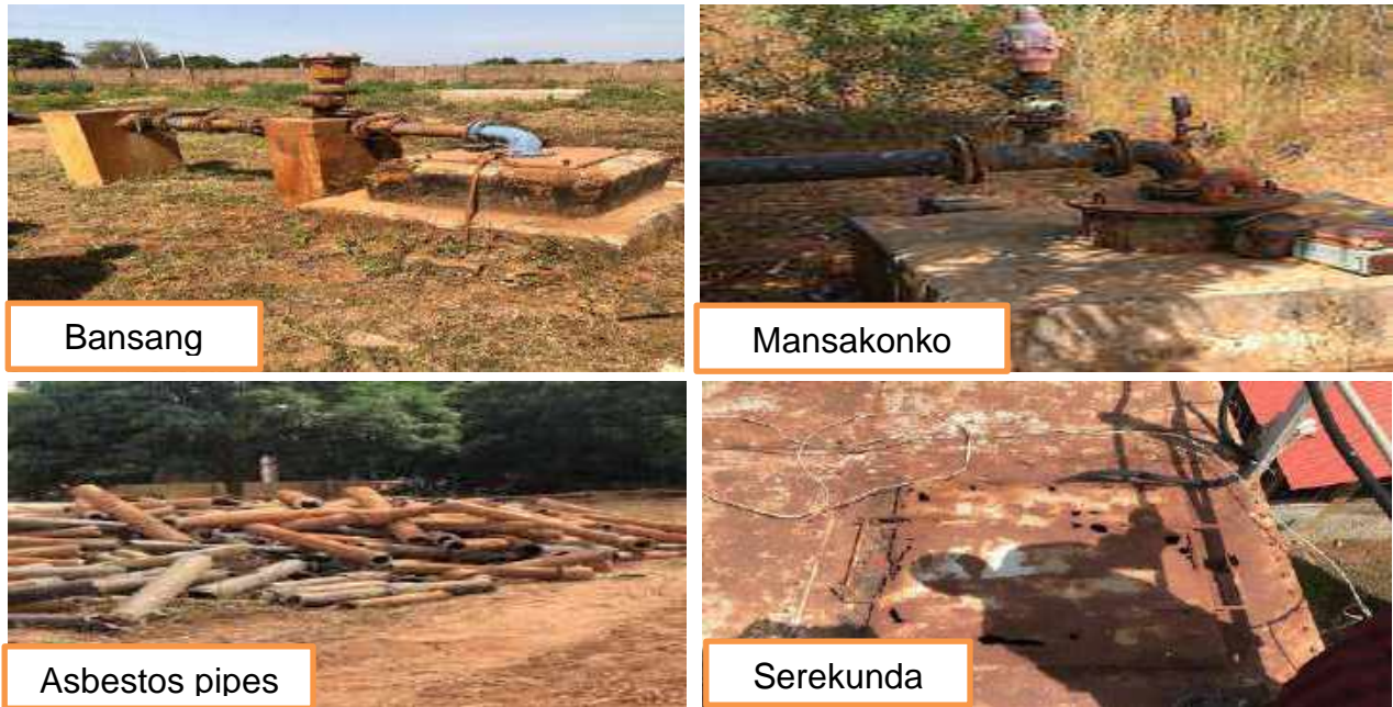
Picture 6: Corroded boreholes at Bansang water facility (top left) and Mansakonko (top right), some of the replaced asbestos pipes placed at Faraja water treatment plant and reservoir at Serekunda water treatment plant (bottom right)
