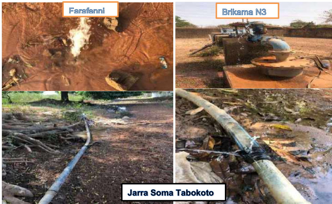
Picture 3: Burst pipes in Farafenni (top) and Mansakonko (down)
