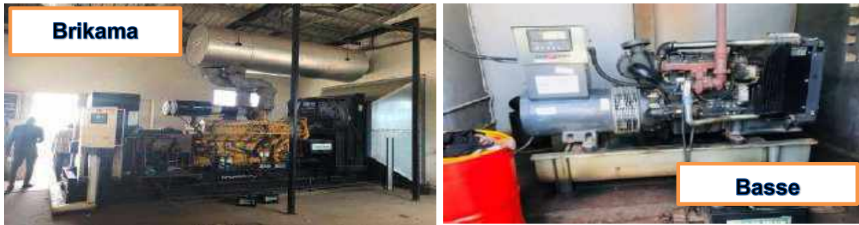
Picture 5: Non- functional Standby Generators at Brikama and Basse water treatment plant.
