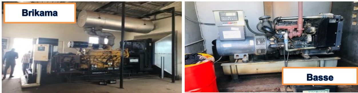
Picture 5: Non- functional Standby Generators at Brikama and Basse water treatment plant.
