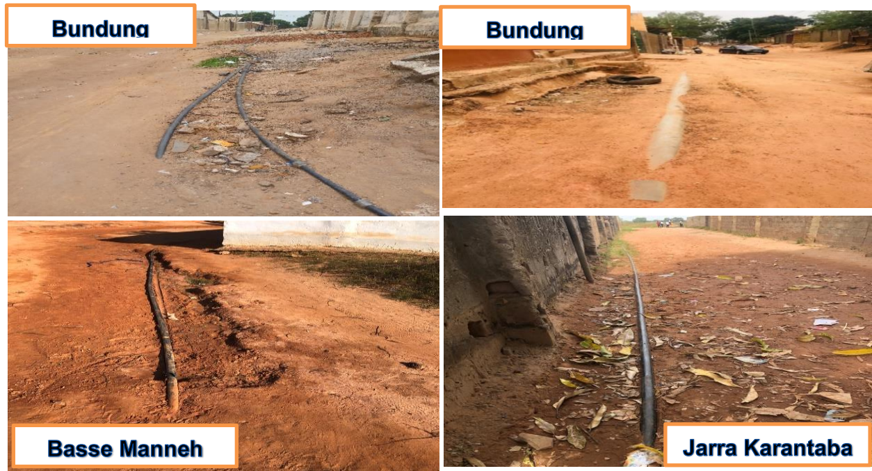
Picture 4: NAWEC’s exposed distribution pipe (top Left), main pipe (top right) in Bundung and exposed distribution pipe (Bottom left) exposed distribution pipe at Jarra Karantaba (Bottom right)
