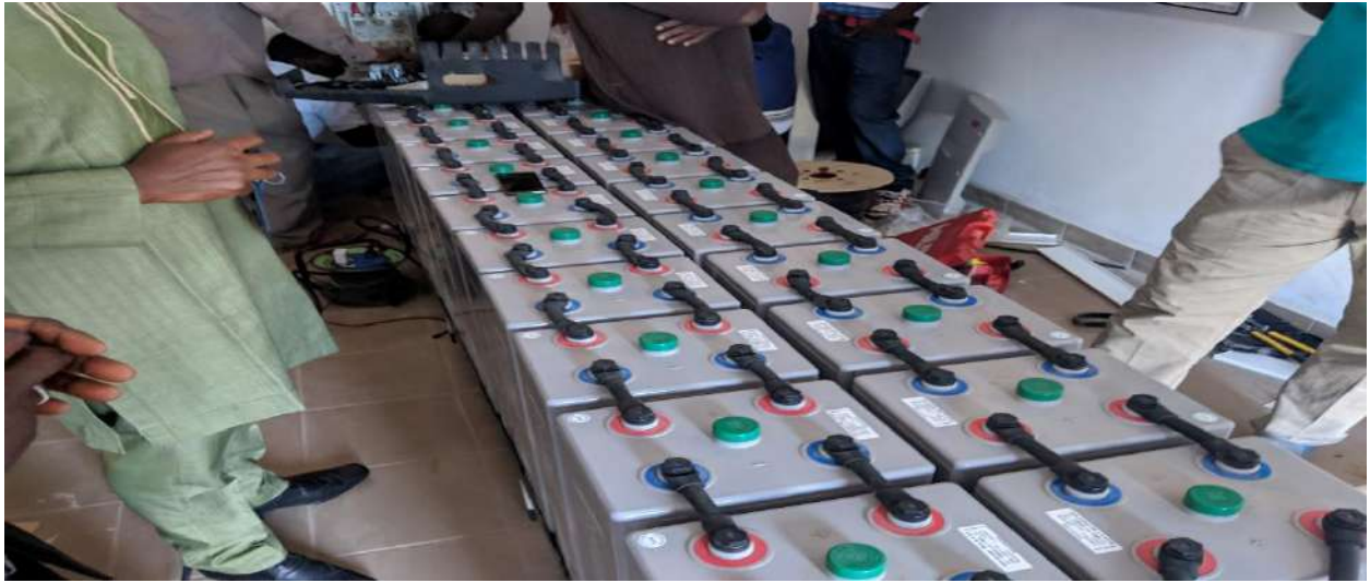
IGPISP: Handing Over of Renewable Energy Equipment to GCCI
